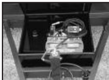
Pump and Battery Box
